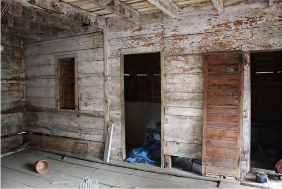
Interior east wall, showing shuttered counting room window, retail room window that was enlarged into a doorway, and half of the double-leaf main entrance door. Photo by Jennifer Glass.
