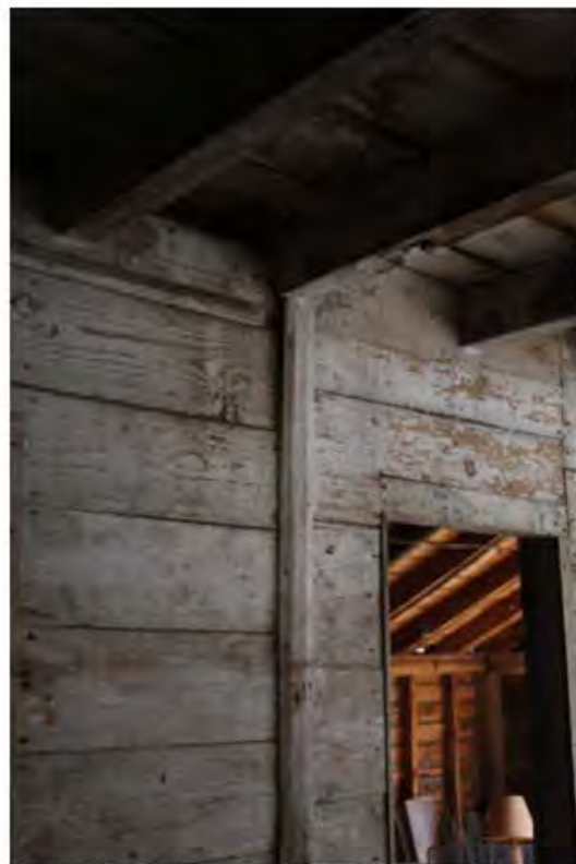
Interior siding join between retail and counting rooms. The beveled board shows partition location; siding to the right is original, and that to the left was installed later. Photo by Jennifer Glass.
