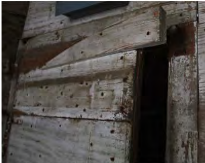
Cleat above counting room door showing lack of original limewash. Photo by Jennifer Glass.
