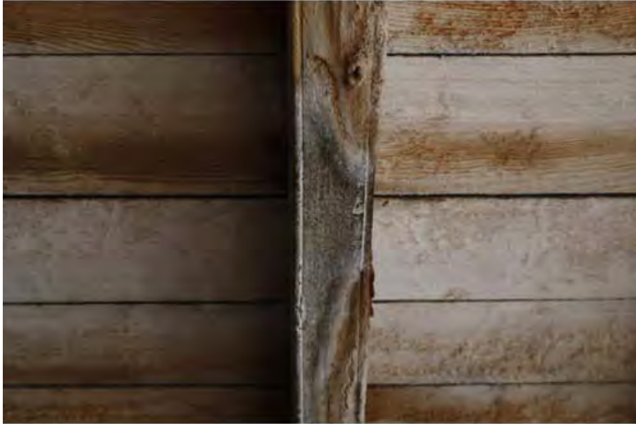
The planed and beaded joists and planed floorboards of the retail room imply that they were intended to be exposed. Photo by Jennifer Glass.
