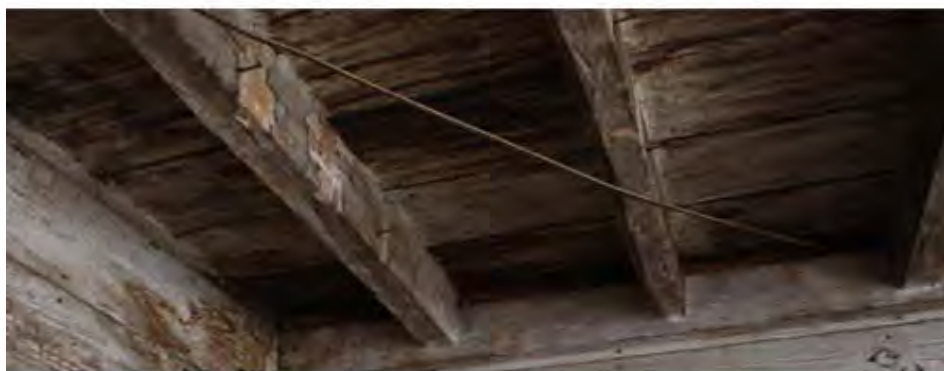
The hewn and pit-sawn joists and the gauged and undercut floorboards of the counting room were probably meant to be plastered. Photo by Jennifer Glass.
